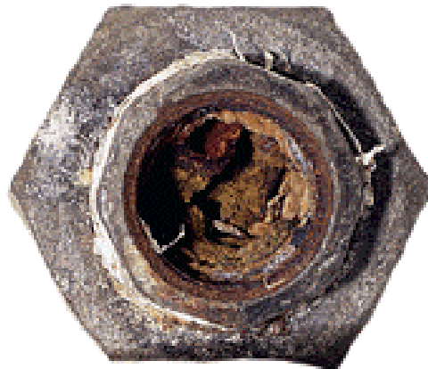
Figure 2-11 Scaling causing pipe blockages
