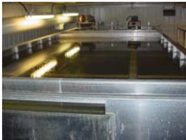
Figure 2-5 A sedimentation tank or clarifier
